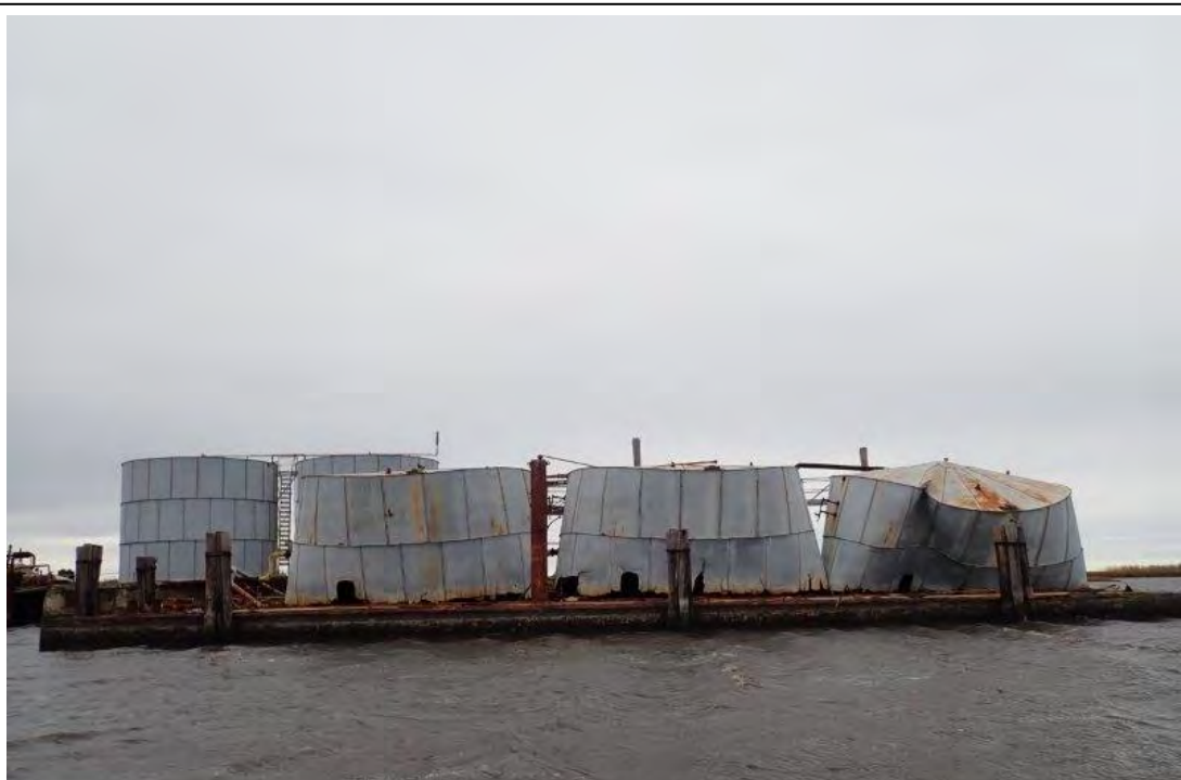
Photograph 114. Site 22: Damaged Oil Field Facility (29°30'39.01"N, 89°59'9.13"W)
