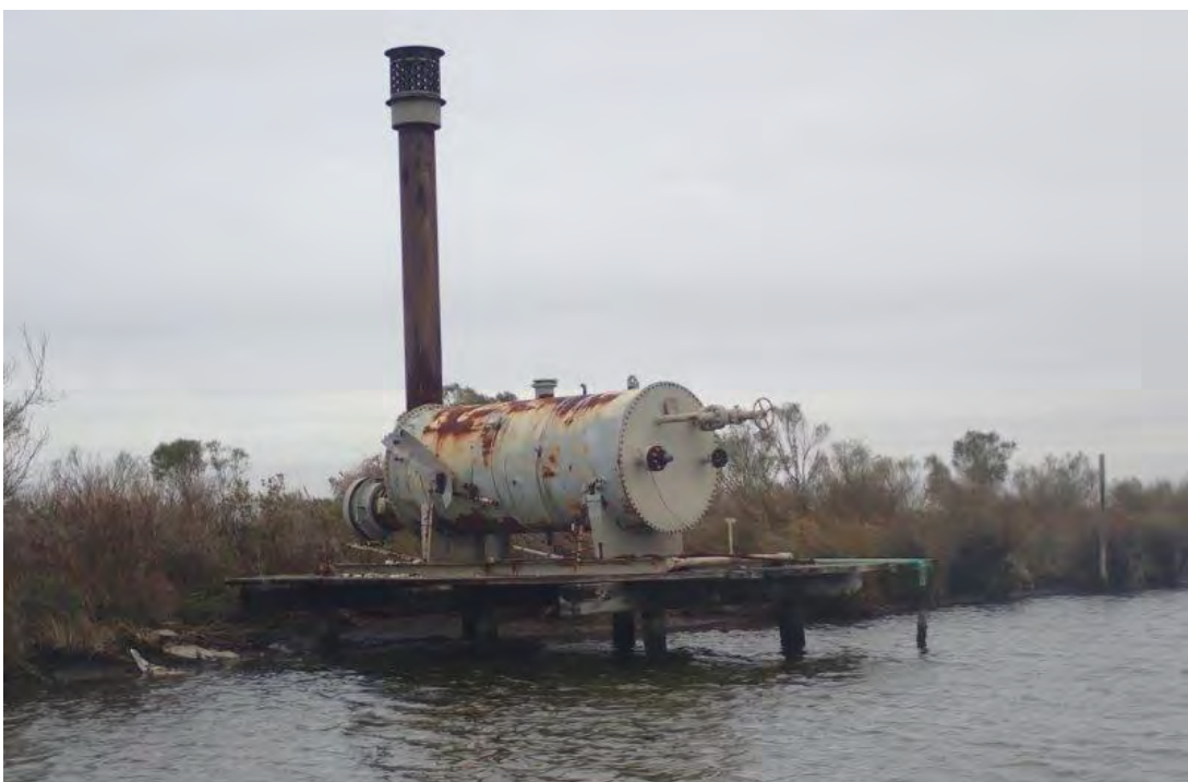
Photograph 144. Site 39: Oil Field Flare Unit
