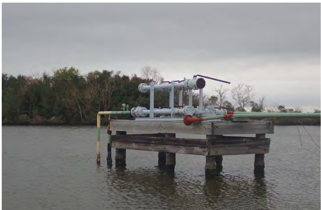
Photograph 146. Site 41: Oil Field Valve Platform (29°35'44.26"N, 90°1'49.46"W)
