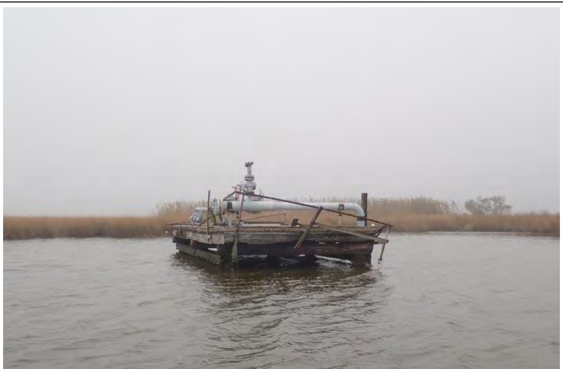
Photograph 102. Site 12: Well Field / Pipeline Valve Site
