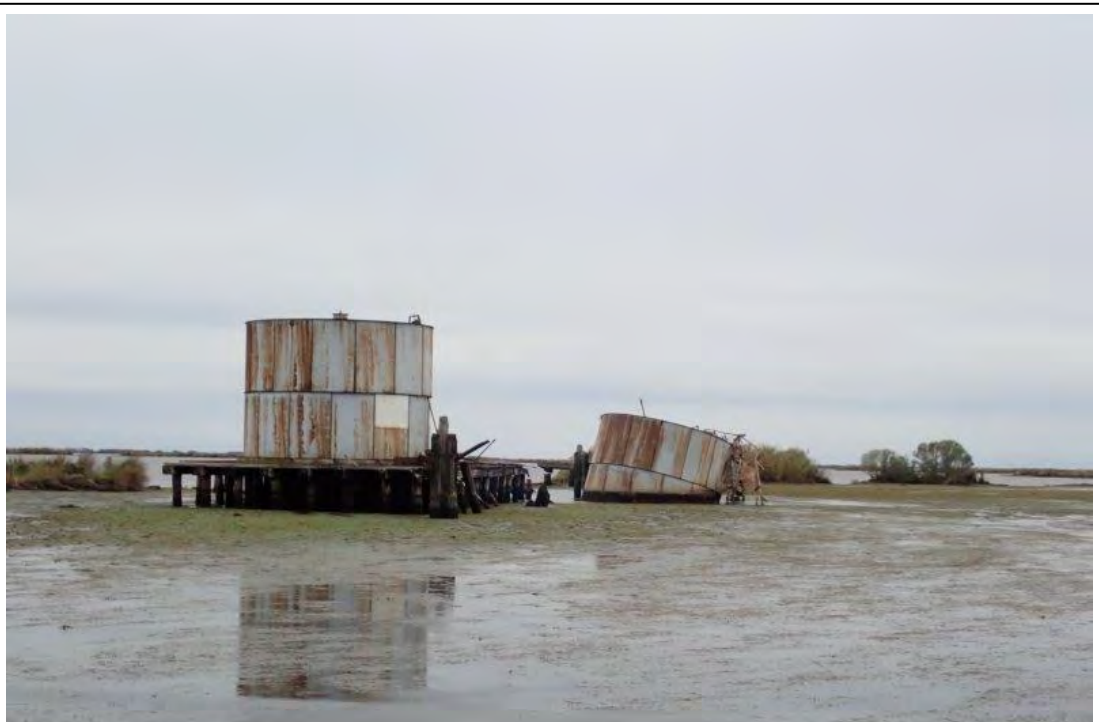
Photograph 86. Site 2: Damaged Oil Field Facility (29°37'7.93"N, 89°59'32.28"W)
