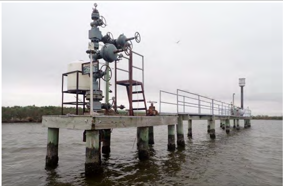
Photograph 139. Site 35: Well Platform with Flare Unit (29°36'40.16"N, 90°3'13.17"W)
