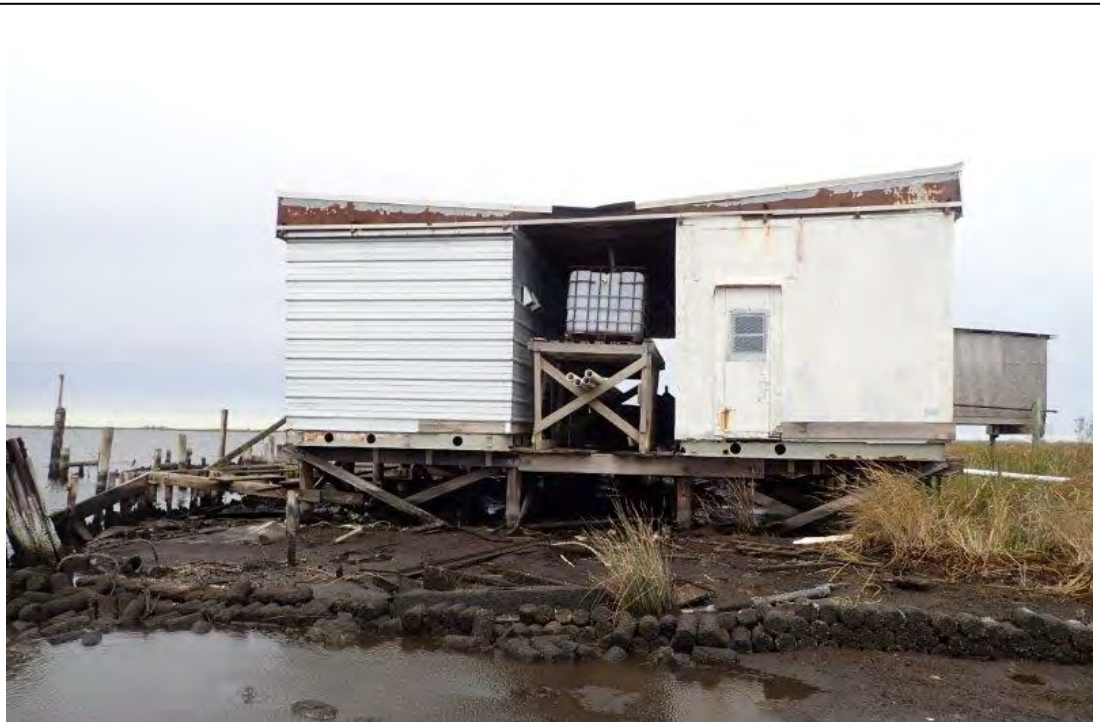
Photograph 90. Site 3: Damaged Camp (29°36'26.76"N, 89°58'46.52"W)
