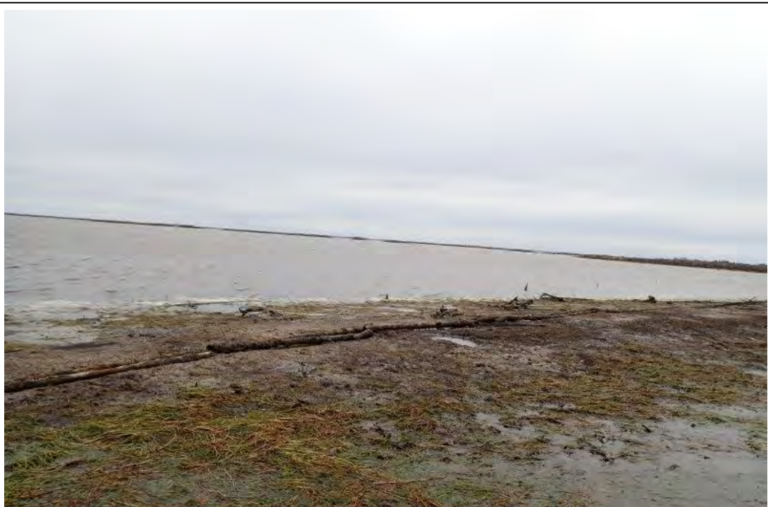
Photograph 88. Site 2: Damaged Oil Field Facility
