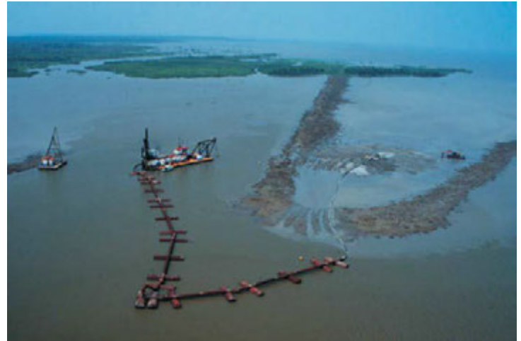
A hydraulic dredge pumps sediment to create new wetland habitat in the project area south of Morgan City.
