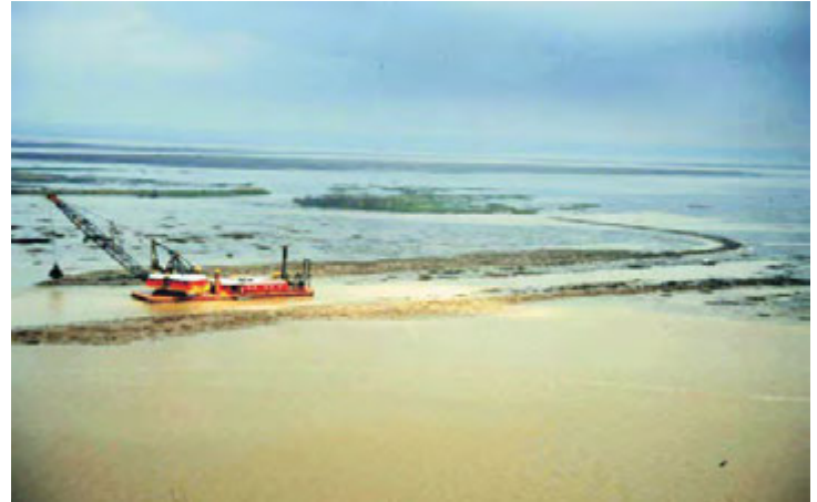
A bucket dredge is shown removing sediment from a shoaled-in channel in order to help reestablish water and sediment flow within the Atchafalaya Delta.
