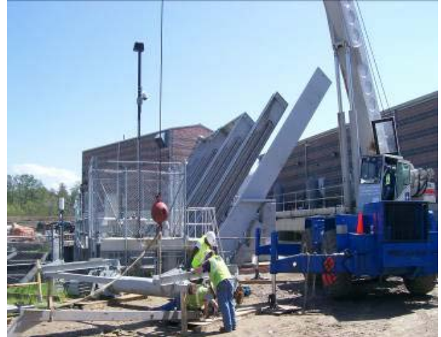
Climber Screens at Westminster Pump Station
