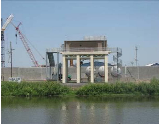
Safe House at Hero Pump Station
