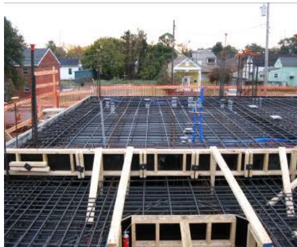
Construction of a Generator Building at the Carrollton Water Treatment and Power Plant Facility
