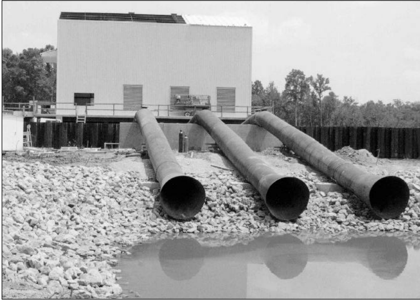
The pump station discharge lines are poised to pump local storm water into the ponding area.
