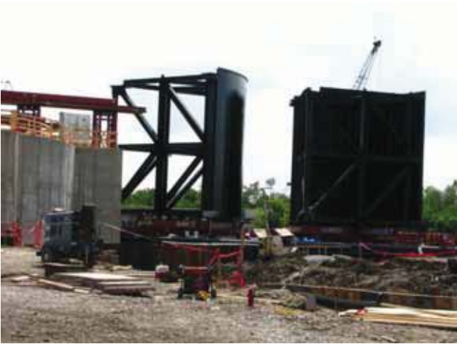
A gantry crane (red, left) moves the 36-ft tall sector gate leaves into place on the Caernarvon Canal. High resolution images are available upon request.
